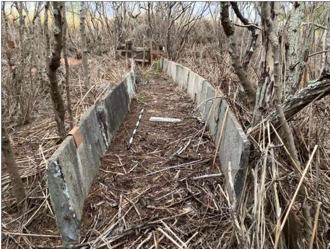
Figure 51. Site 7346 Feature 155-D, western portion of intact flume alignment, view to the west.
