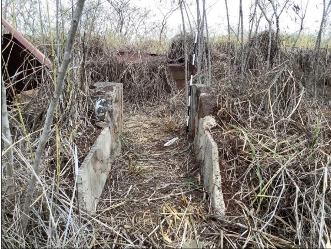
Figure 54. Site 7346 Feature 155-E, sluce outlet that formerly released water into Feature 155-F, view to the northwest.
