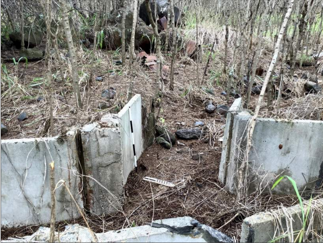
Figure 70. Site 7346 Feature 155-M, sluice gate indicating the presence of a former western flume branch at the northern end of the southernmost section, view to the southwest.
