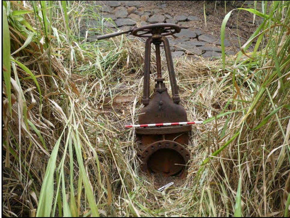
Figure 26. Wheel-operated sluice valve located at the dam base; view to the northwest.
