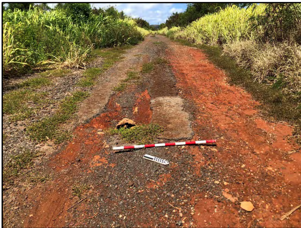
Figure 22. Overview depicting deteriorating paved segment of railway alignment.
