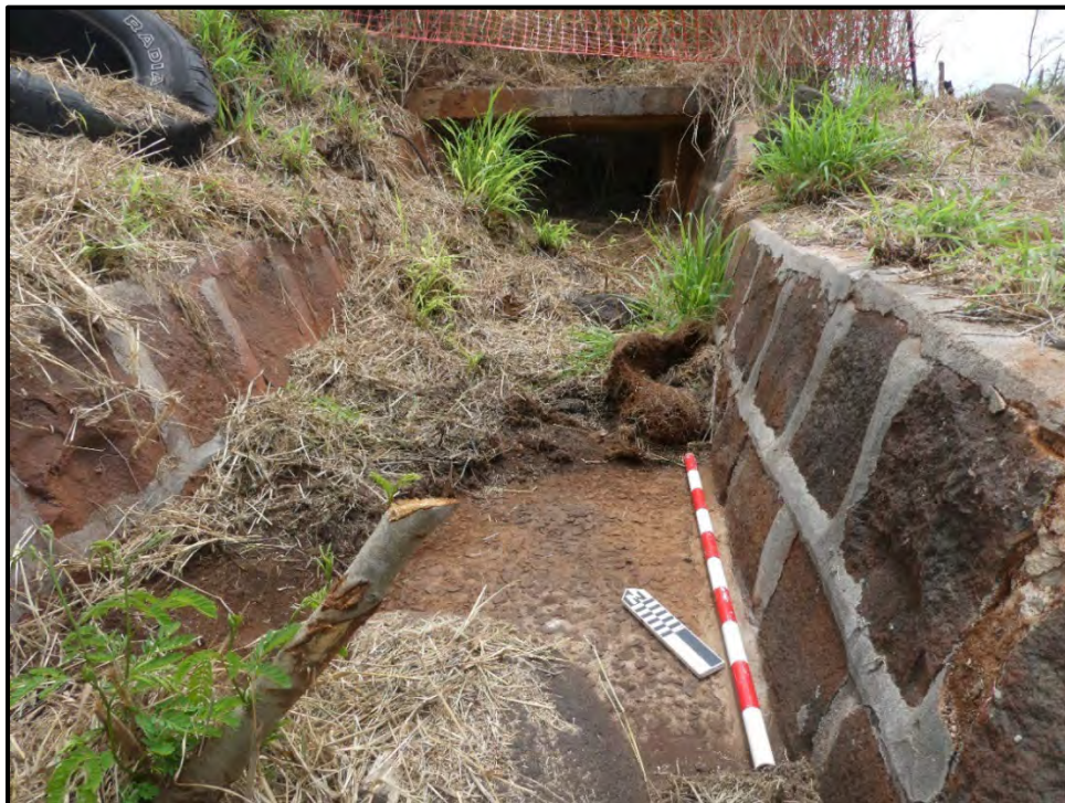
Figure 18. Irrigation ditch segment detail showing rock-lined canal with box culvert in the background; view to the north-northeast.
