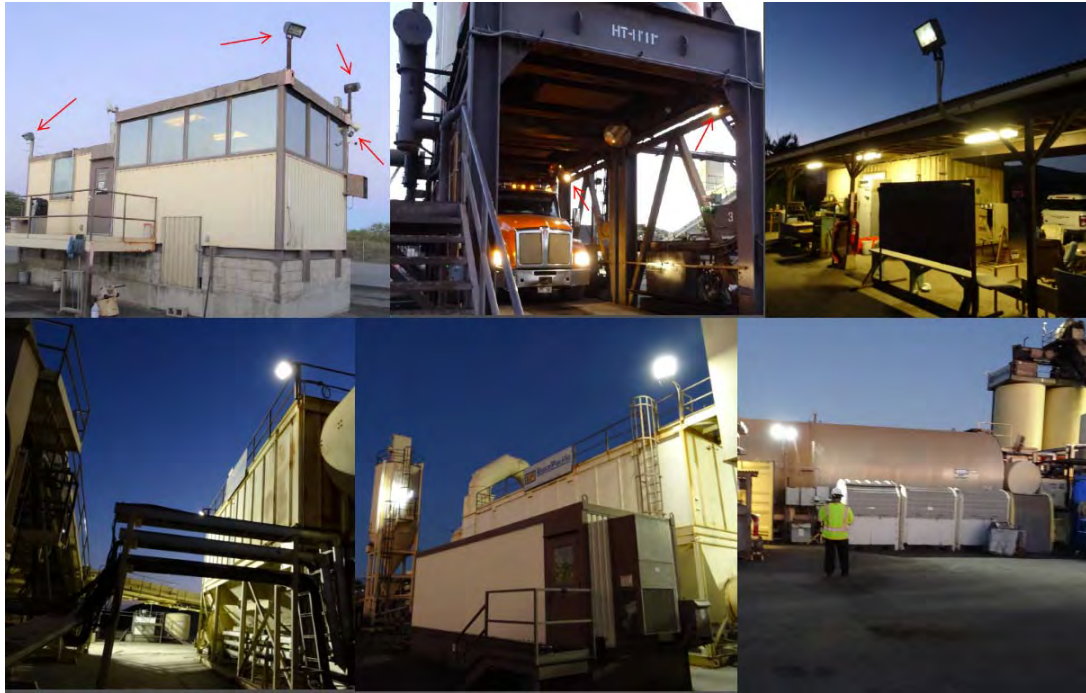
Figure 4 – Asphalt Batching Plant - Various light fixtures. Clockwise from upper left: Various floodlights on the operations building; bare bulb light fixtures; HID Floodlight (top) and fluroescent wraparound light fixtures at the QC lab; LED floodlights; LED floodlight; and fluroescent induction floodlights.
