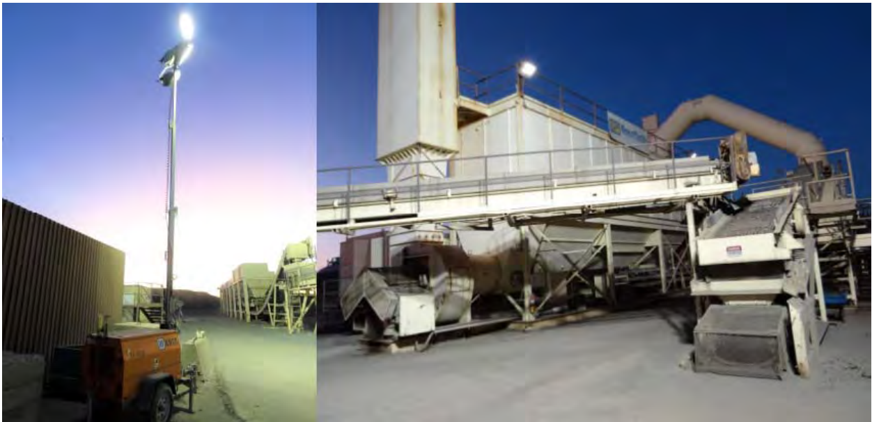
Figure 3 – Asphalt Batching Plant - Portable generator lighting system (left); Area illuminated by the portable generator lighting system.
