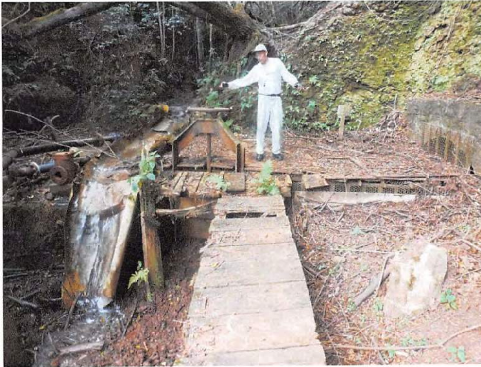
Metal flume diverting water from Waiahole Ditch to the intake.
