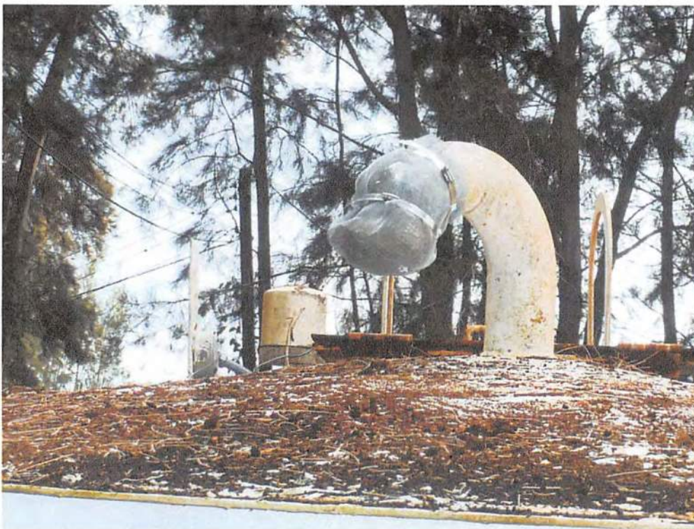
Air vent on head tank properly screened and downturned.
