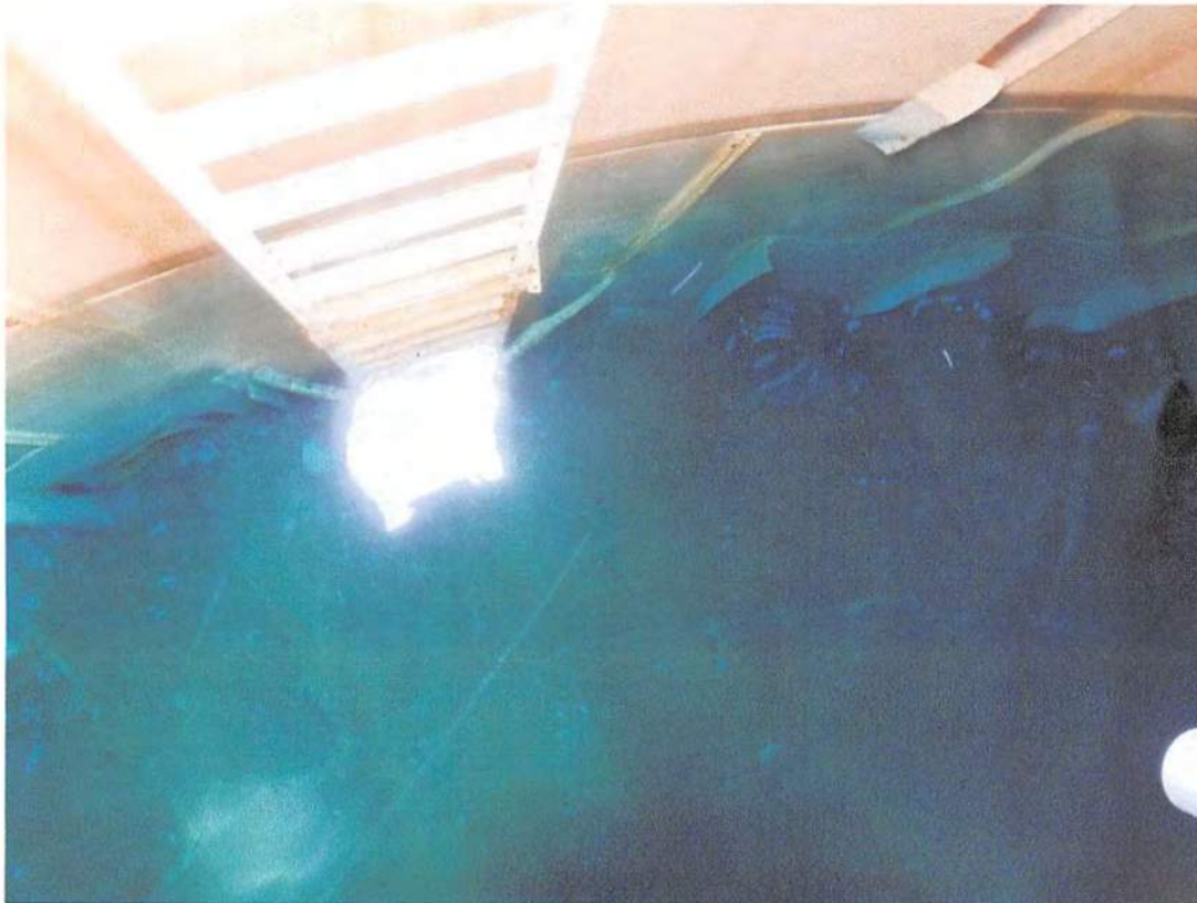
There is particulate in the water, most likely the paint that has been falling off the ladder and access hatch due to rust.
