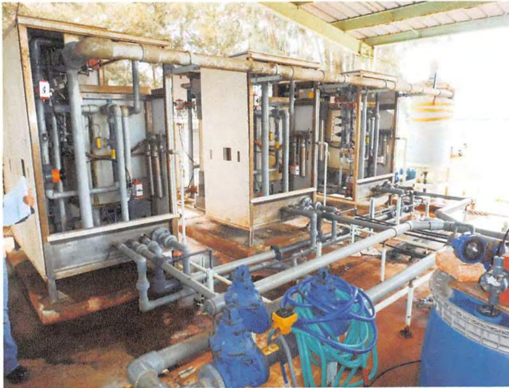
Three Memcor microfiltration units, exposed to the elements without proper enclosure.
