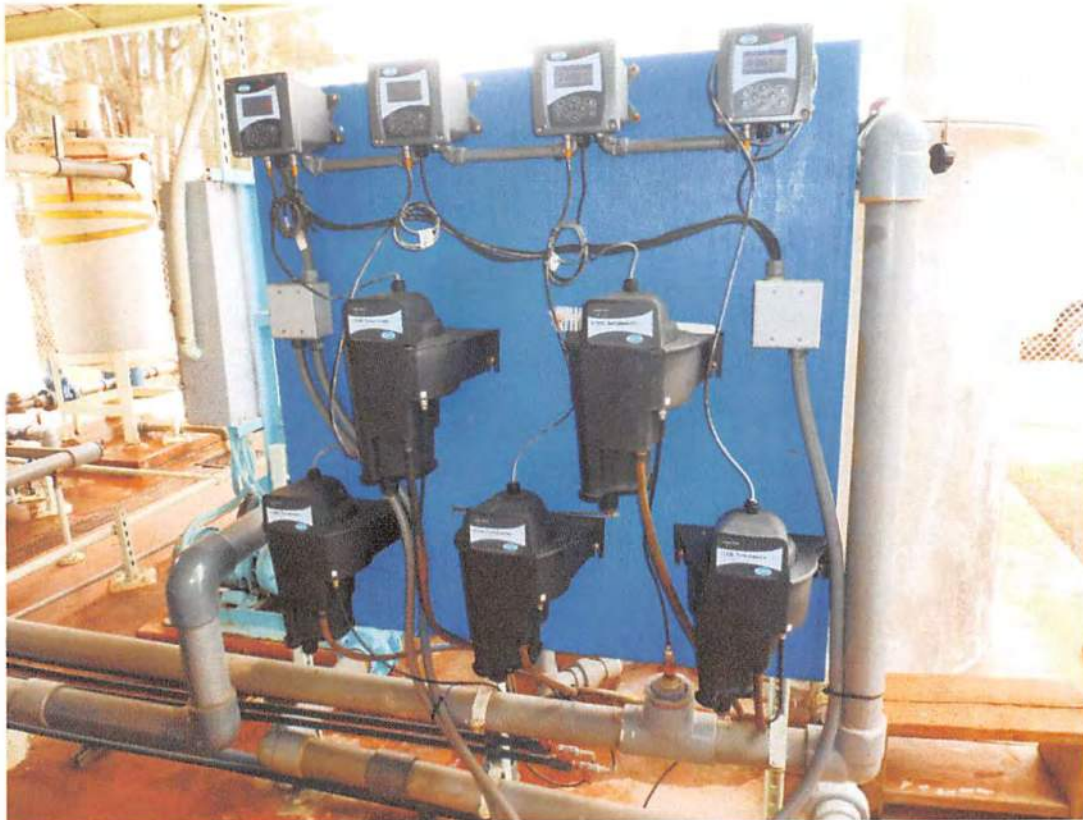
Turbidity monitors at water treatment plant.
