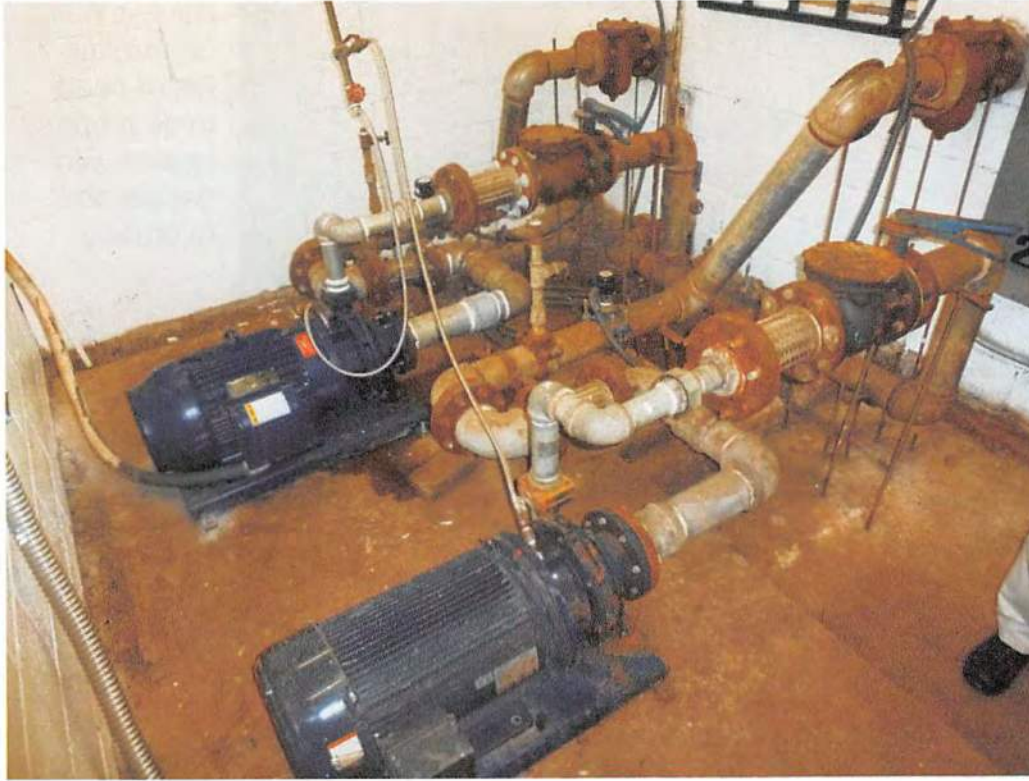
Pumps that boost water to the head tank.
