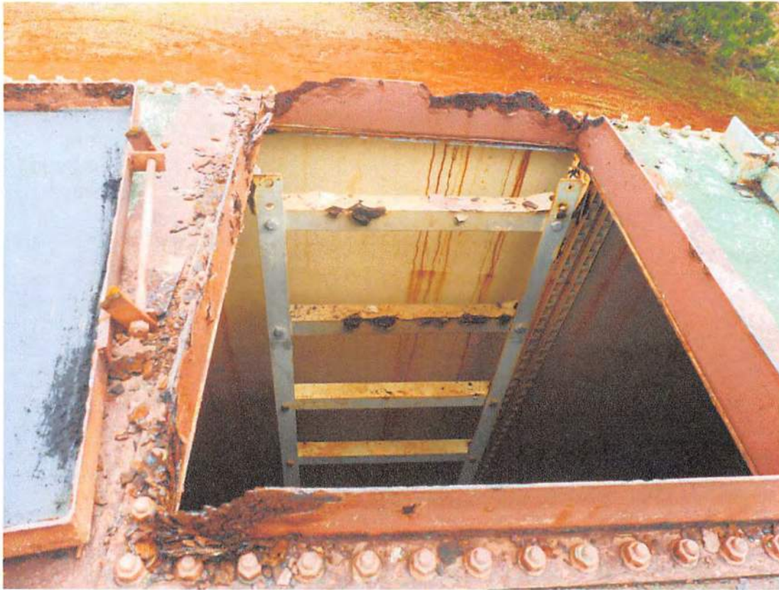
The ladder leading into the tank from the access hatch is rusty and peeling paint has been falling into the water.
