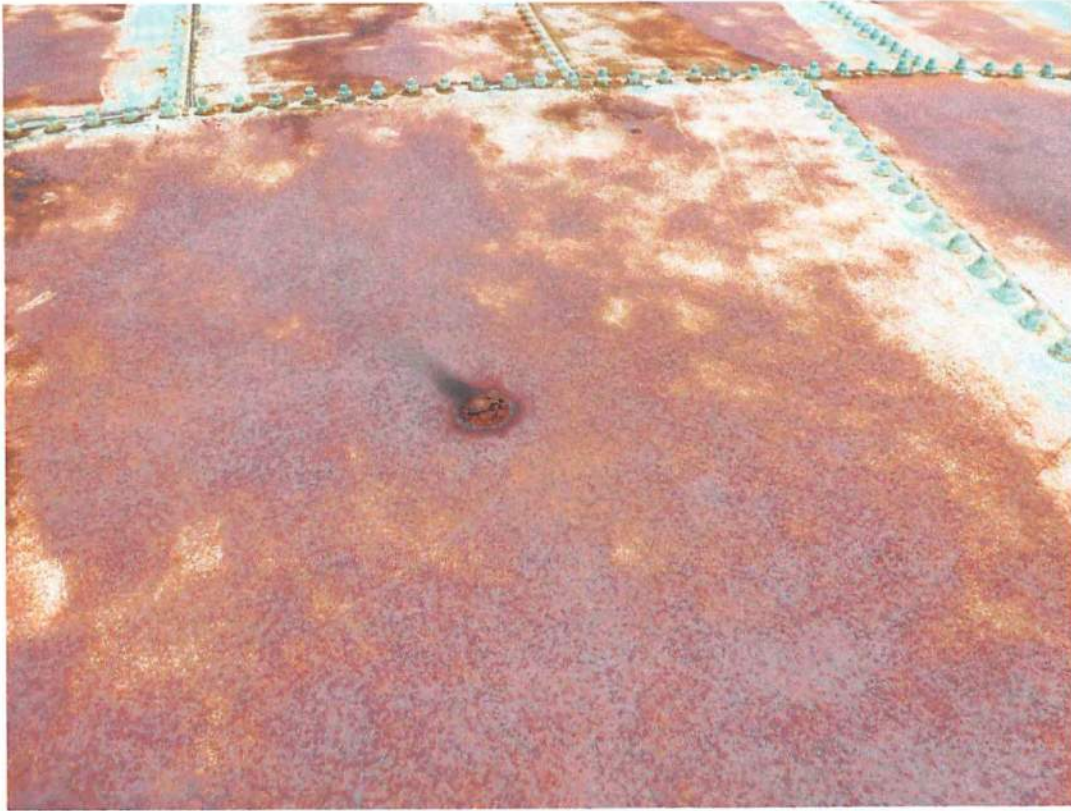
The clearwell roof is very rusty and blisters have begun to form.
