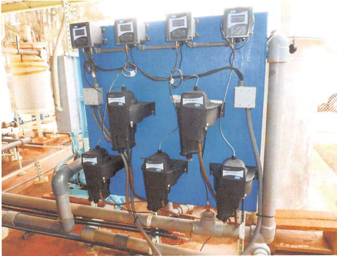
Turbidity monitors at water treatment plant.
