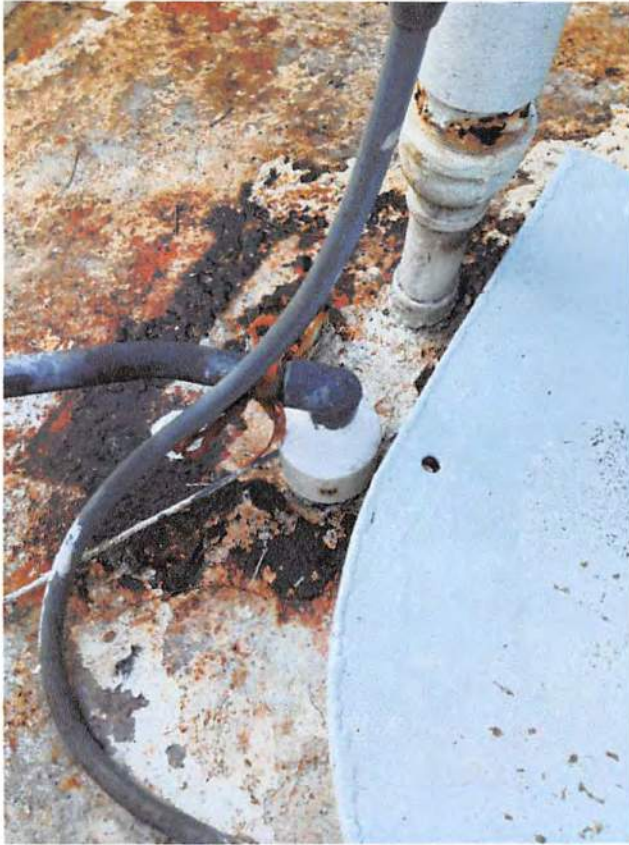
Influent line to the raw water tank.
