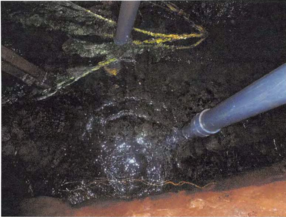
Water system intake.
