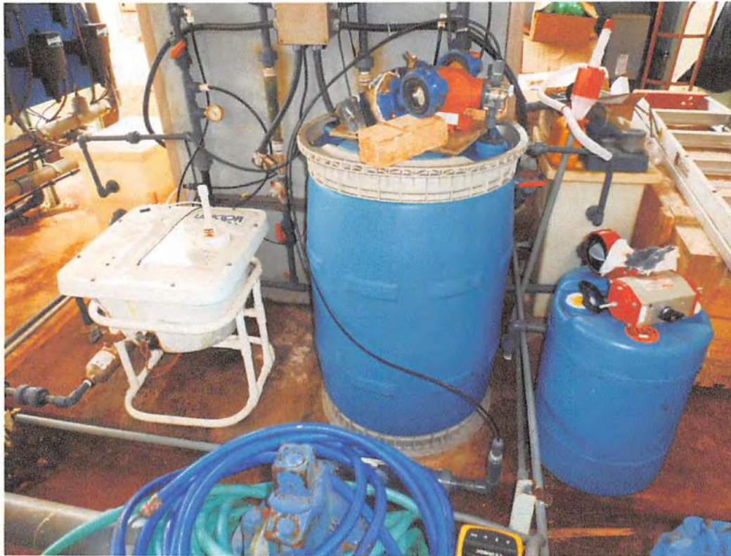
Hypochlor barrel for on-site disinfection.
