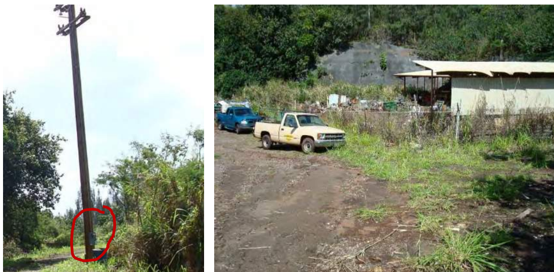
Figure 1: Existing HECO meter is located on site, next to the abandoned storage bldg
