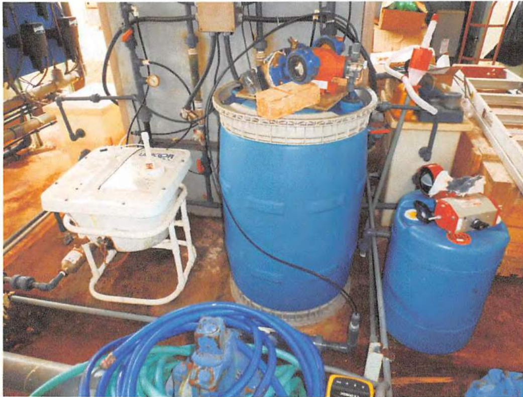
Hypochlor barrel for on-site disinfection.
