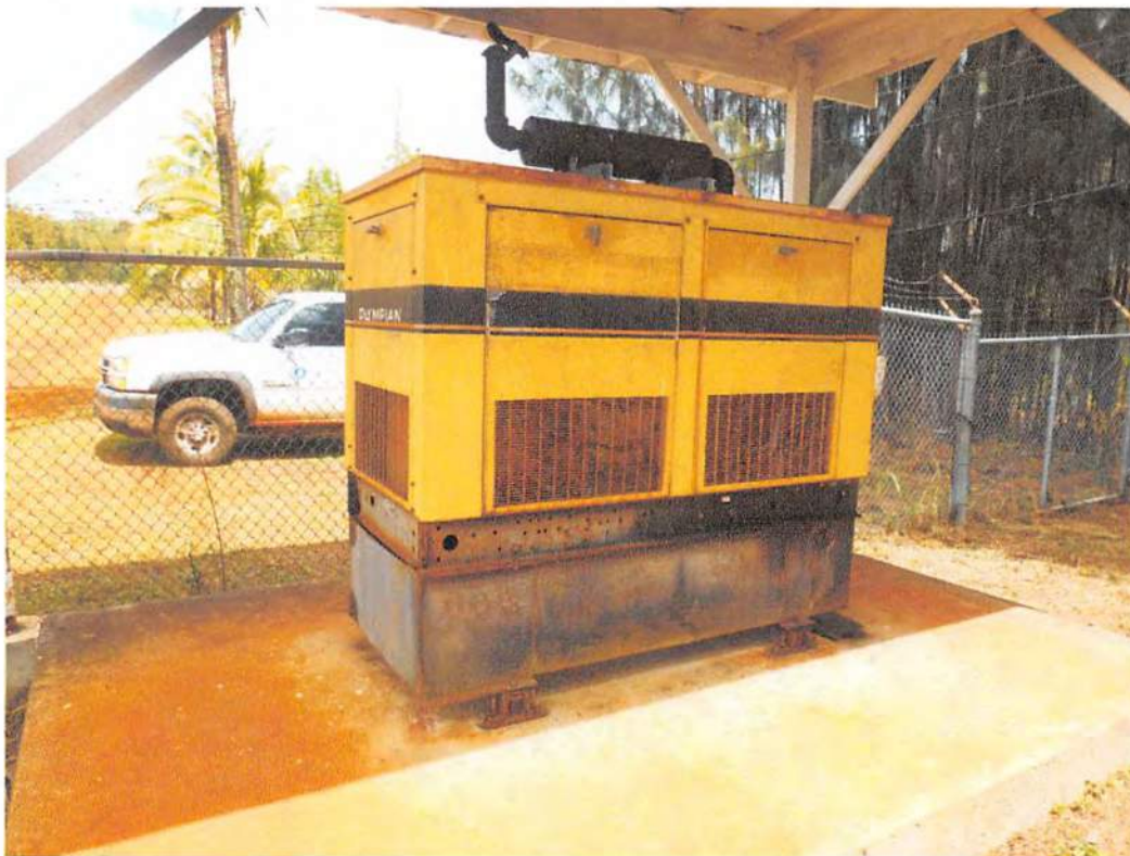
35kW generator for backup power.
