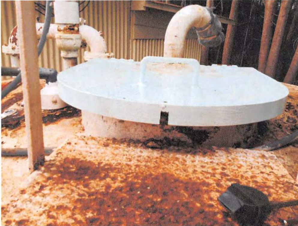
Access hatch on the raw water head tank, properly sealed with gasket and overhang.
