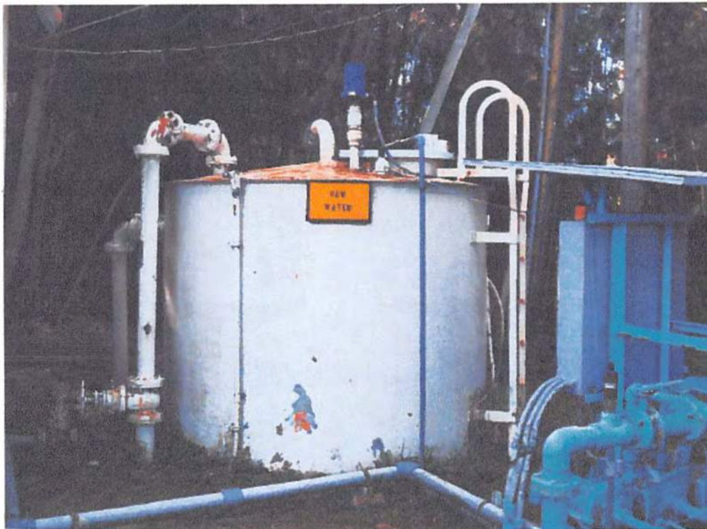
Head tank next to the water treatment plant.
