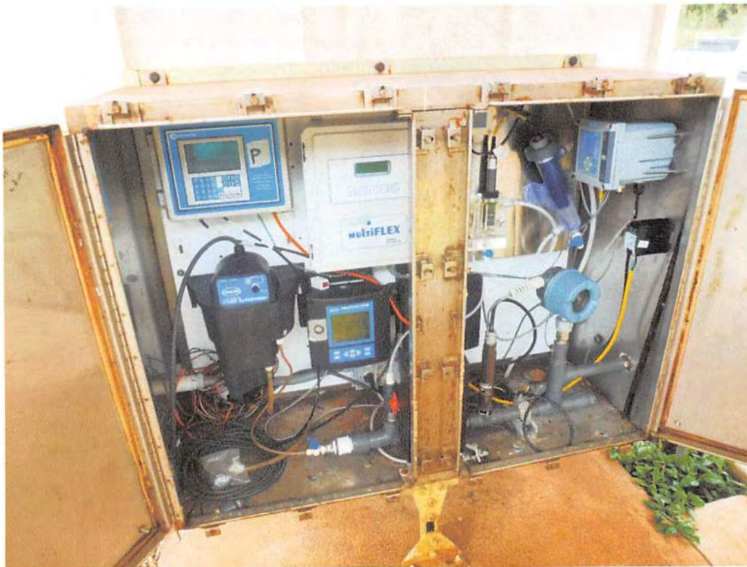
Monitors in an enclosure at the clearwell site.
