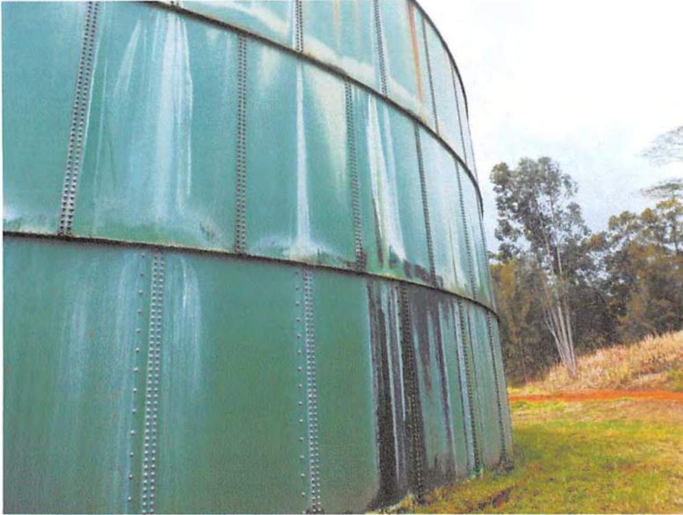
The clearwell is leaking significantly at the joints.
