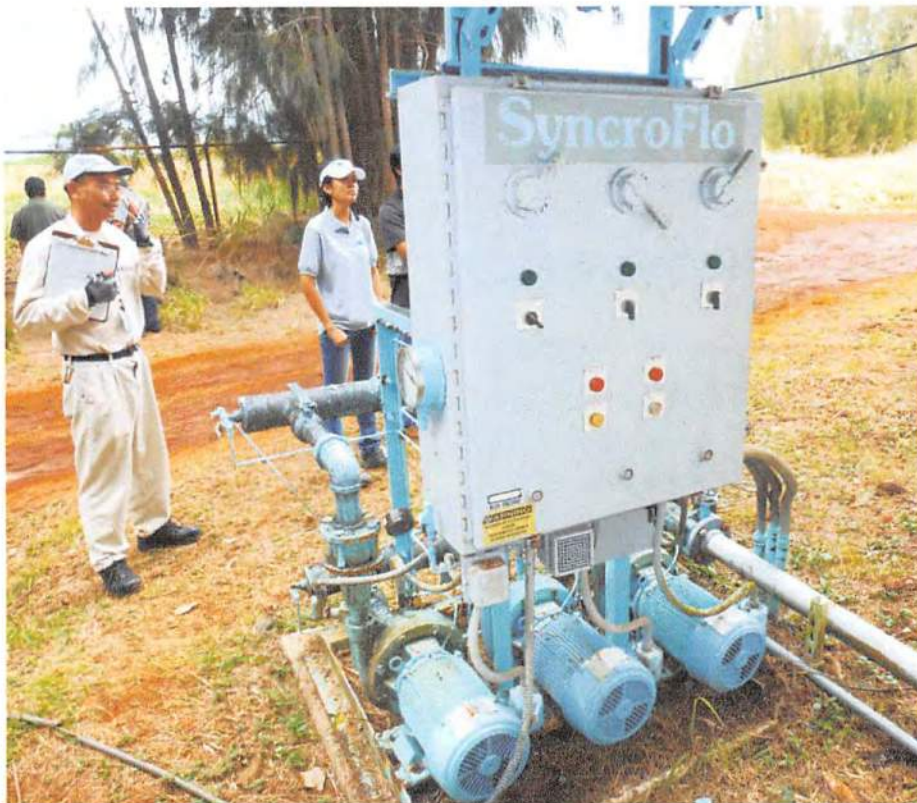
Three booster pumps to run water from the head tank to the water treatment plant.
