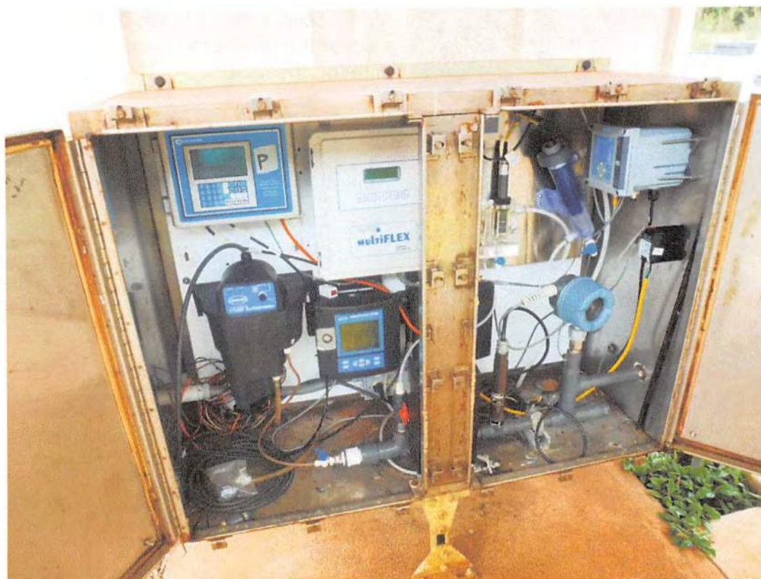
Monitors in an enclosure at the clearwell site.
