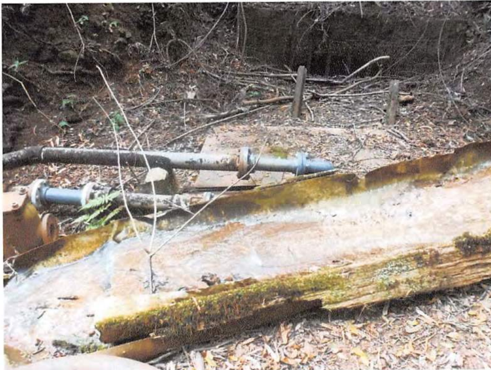
Metal flume diverting water from Waiahole Ditch to the intake.
