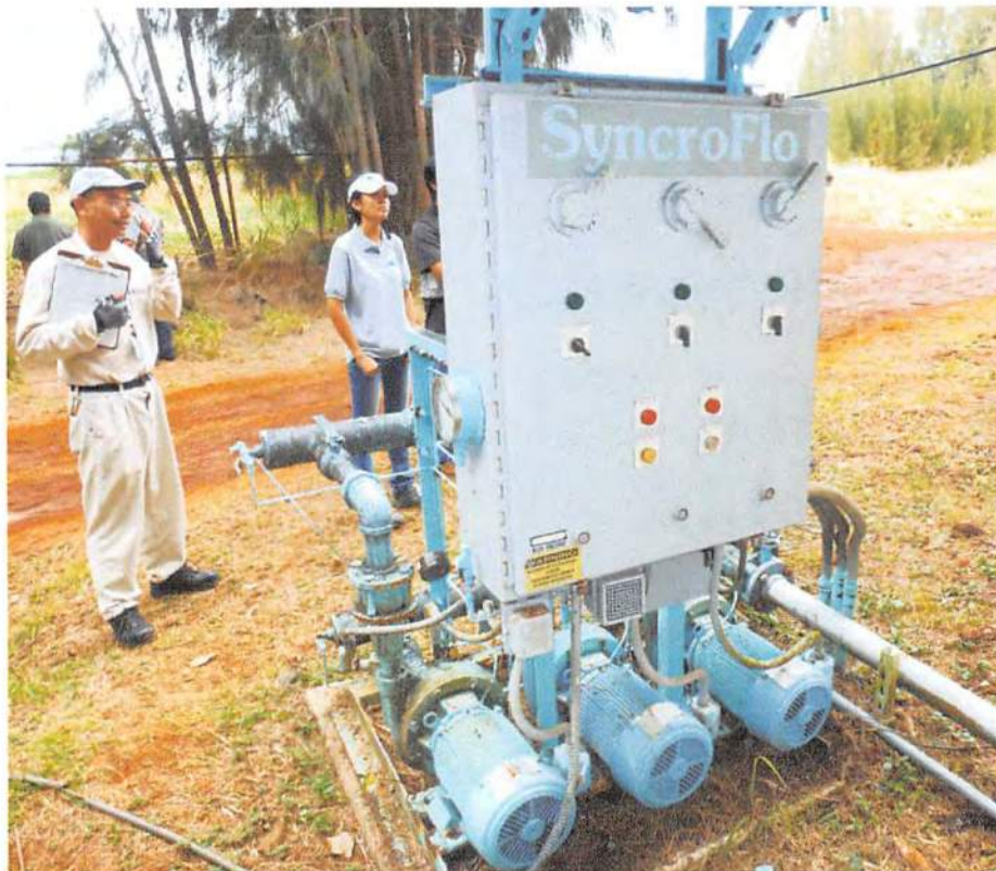
Three booster pumps to run water from the head tank to the water treatment plant.
