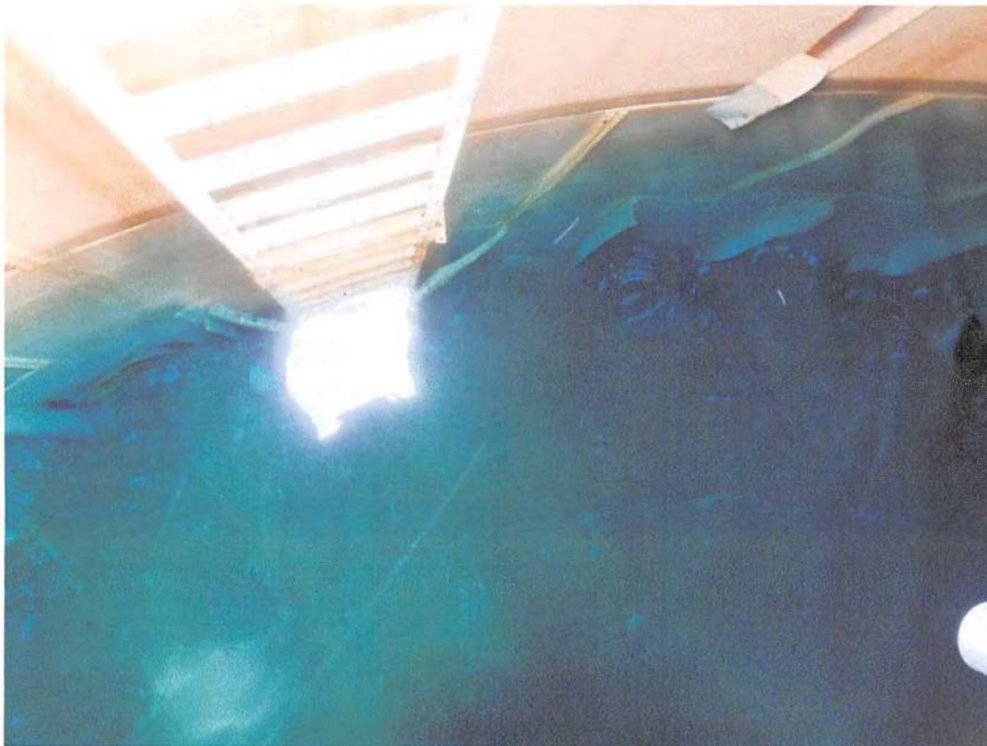
There is particulate in the water, most likely the paint that has been falling off the ladder and access hatch due to rust.
