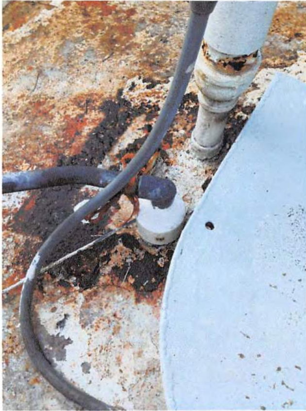
Influent line to the raw water tank.
