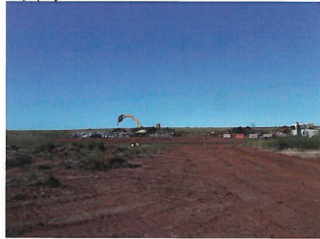
12. Adjoining metal scrapyards with workers actively removing debris.
