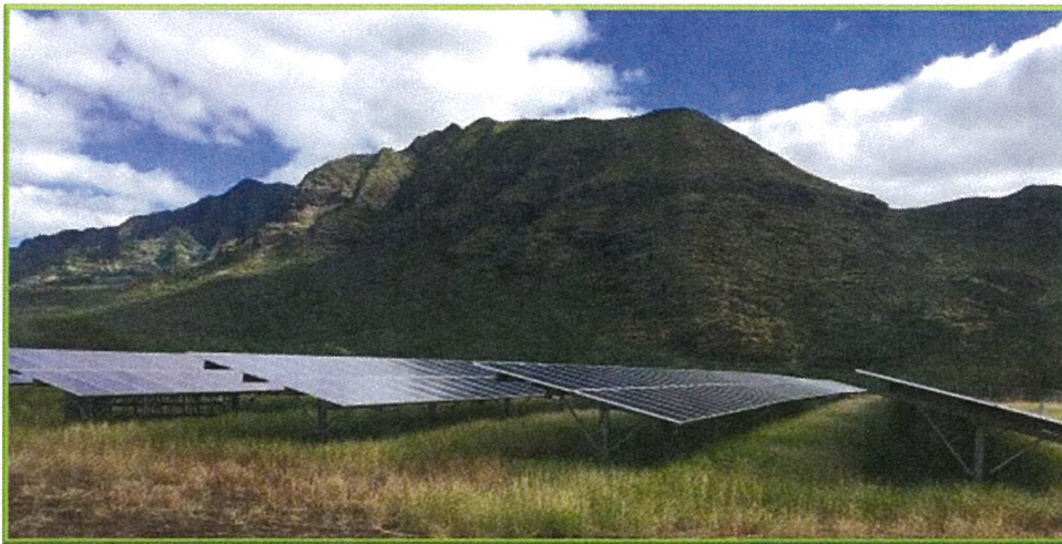
Photovoltaic Panels and Racking System
