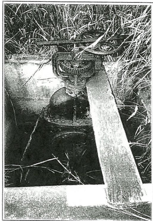
Figure 4: Water Pump in Sugarcane Field. View to West.
