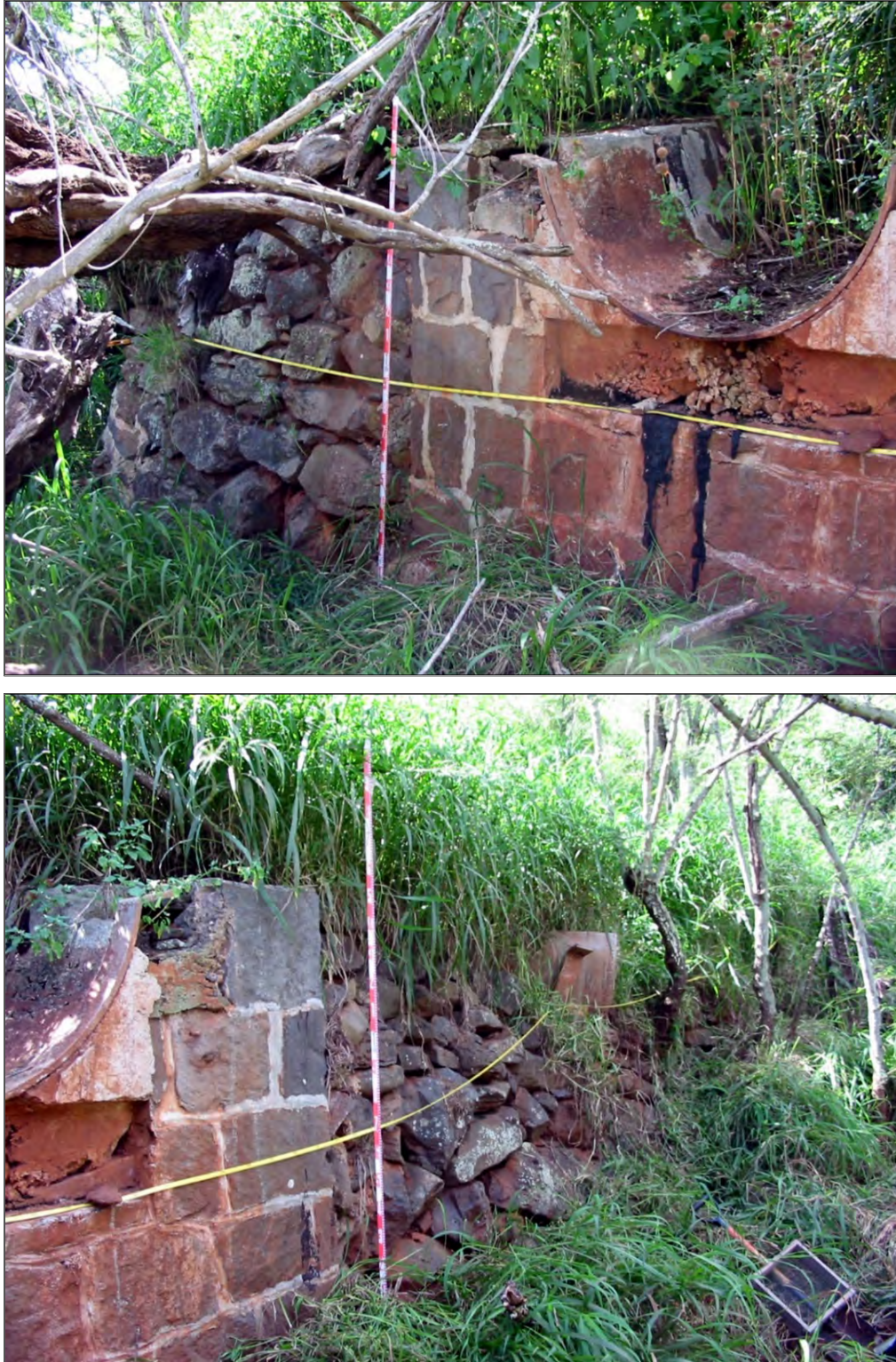
Figure 83. Showing the eastern (top, view to east) and western (bottom, view to south) ends of the southern portion of SIHP # 50-80-09-2268 Feature A: flume bridge (Tulchin and Hammatt 2004:55)
