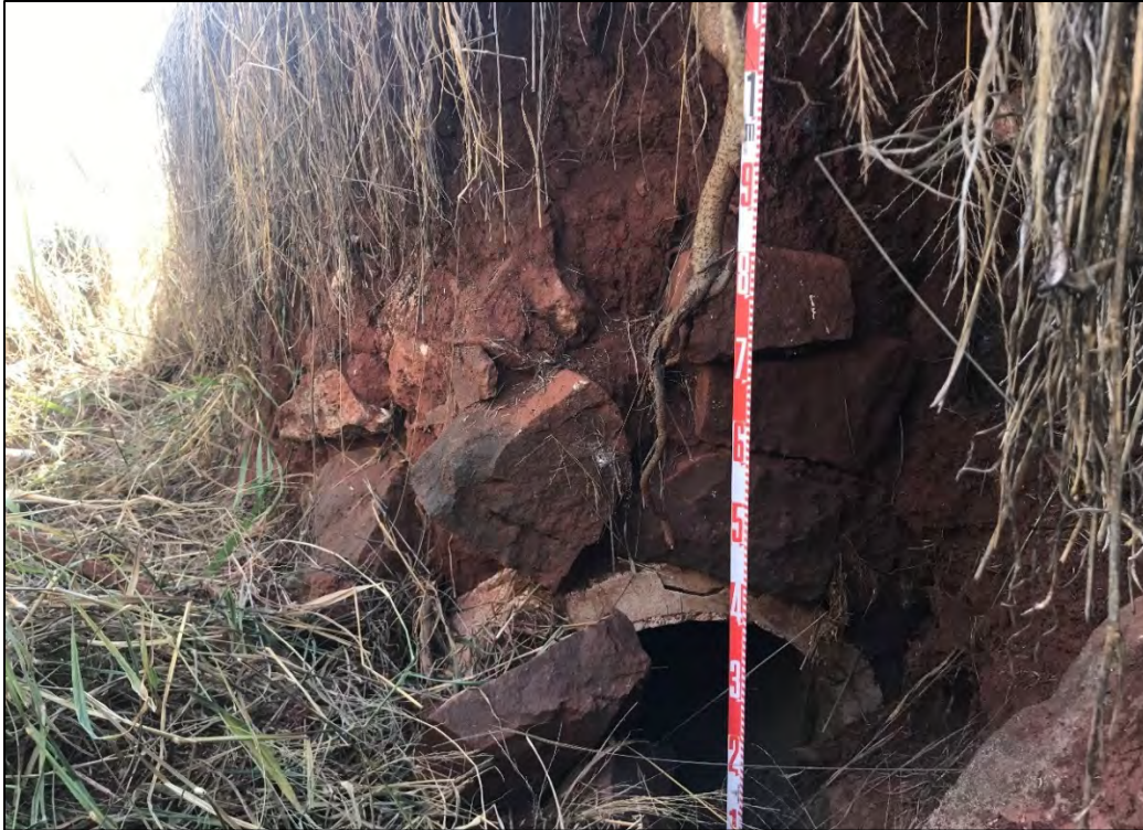
Figure 48. Upper portion of SIHP # 50-80-08-5593 Feature 1 showing concrete pipes, view to east (collapse to the southwest, at right, may have covered the second pipe)
