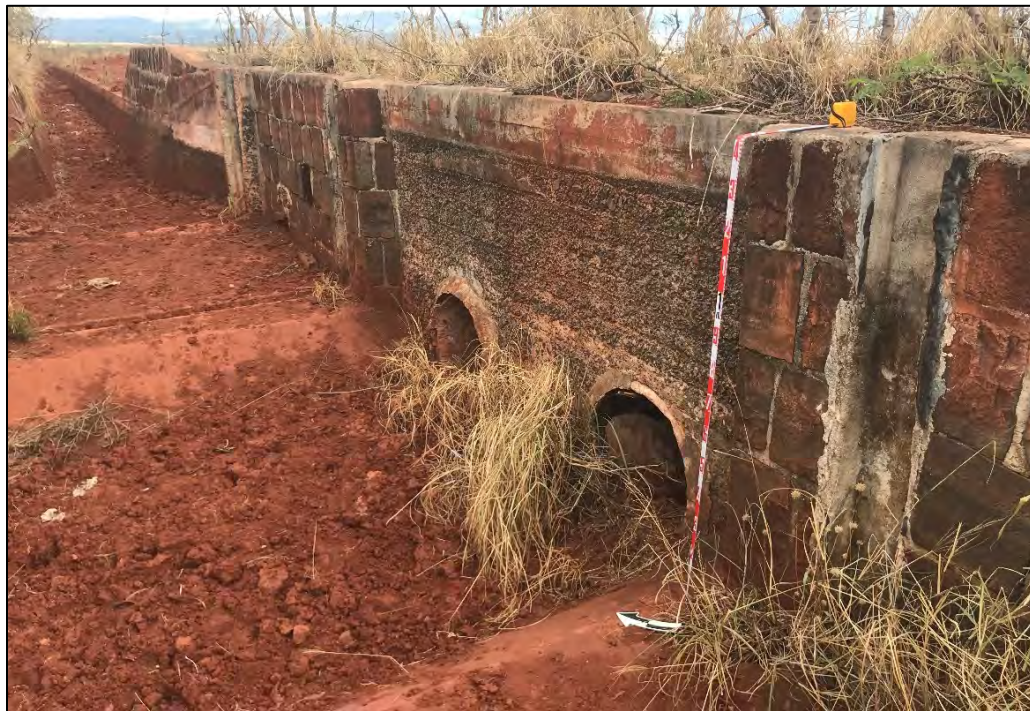
Figure 54. Overview of SIHP # 50-80-08-5593 Feature 2A and SIHP # 50-80-09-2268 Waiahole Ditch portion, with catchment basin (foreground) and drain pipes, view to east
