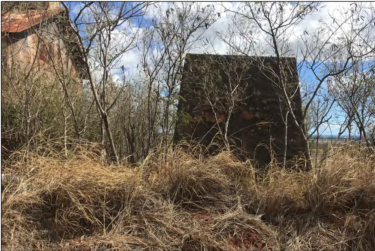
Figure 47. Pump House No. 12, southeast of the project area (mill building to the left), view to southeast
