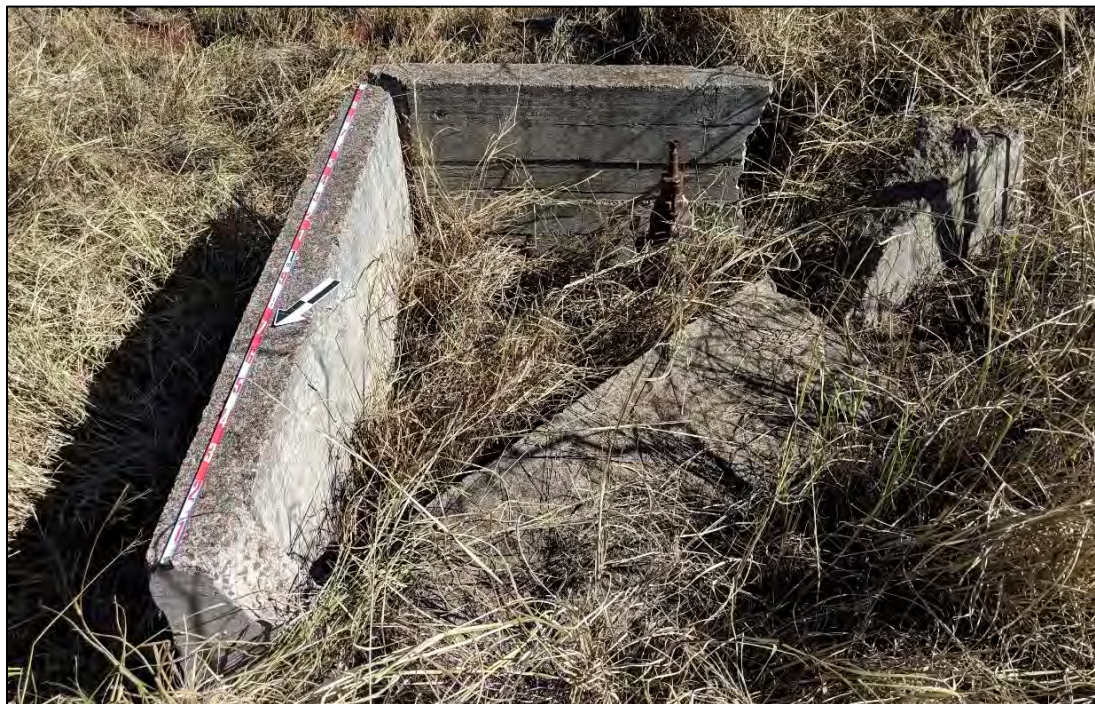
Figure 70. Collapsed walls with pipe, component of SIHP # 50-80-08-5593 Feature 2C, view to southeast
