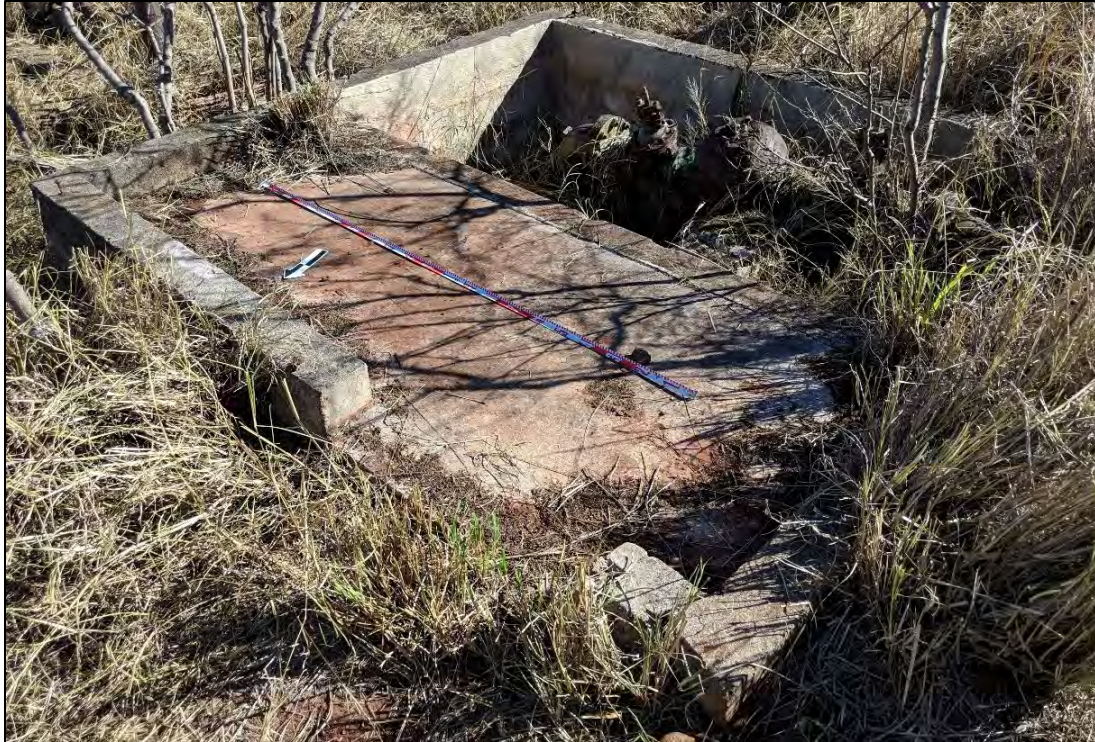
Figure 69. Overview of concrete foundation and pipes component of SIHP # 50-80-08-5593 Feature 2C, view to southeast
