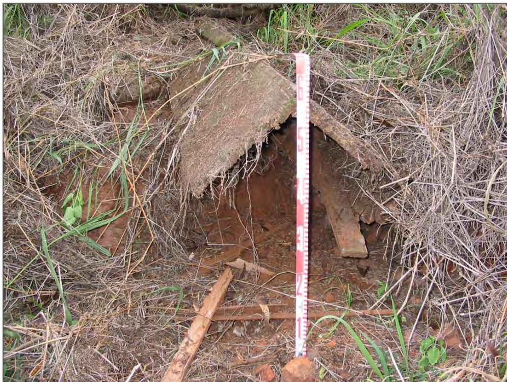
Figure 90. SIHP # 50-80-09-2268 Feature C, showing partially intact wooden flume section, view to south (Hunkin and Hammatt 2009:52)
