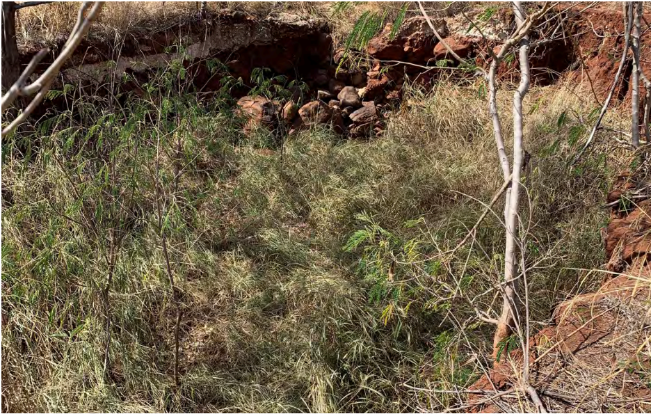
Photo 5. Eroded right bank and bed of Kalio Gulch within the Project Area. 1/31/2019.
