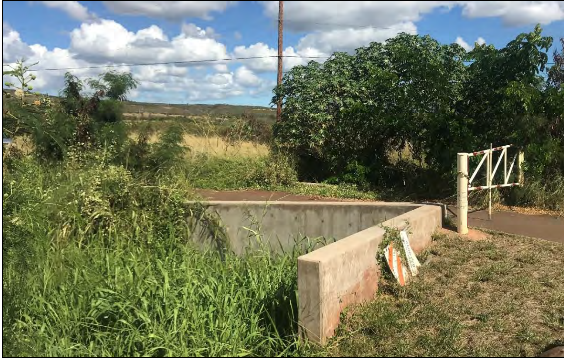
Figure 37. Overview of modern concrete culvert at the base of the access road (junction with Palehua Road), view to northeast
