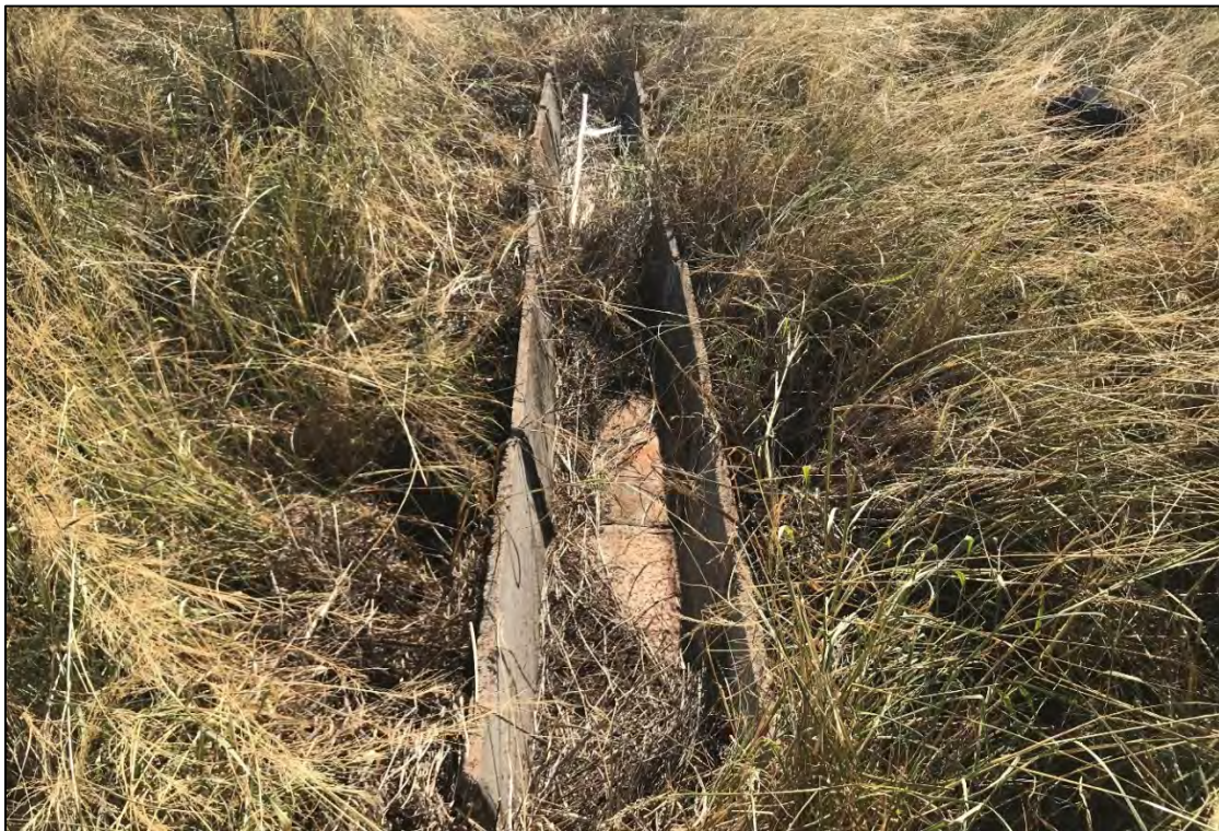
Figure 38. Overview of concrete flume in central northern project area, view to southeast
