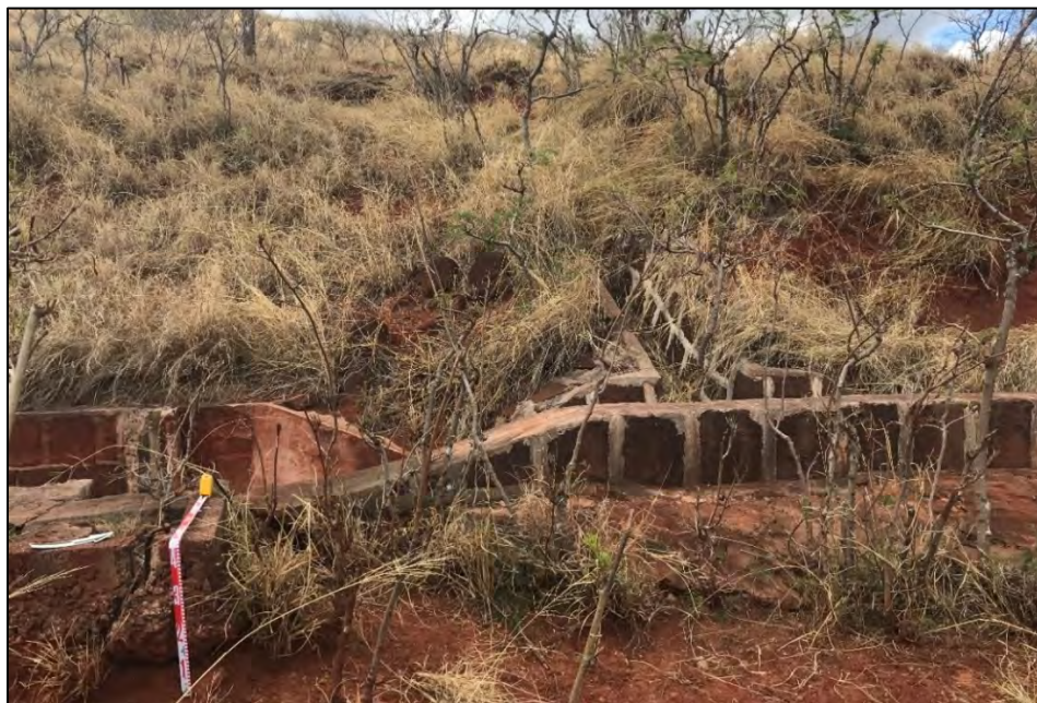
Figure 59. Overview of SIHP # 50-80-08-5593 Feature 2A complex with eastern flume (right), extending into SIHP # 50-80-09-2268 Waiahole Ditch, view to northwest
