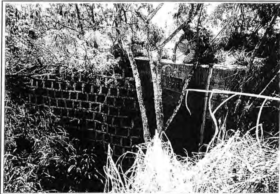
Figure 6: Irrigation System Bridge. Note Date of 1928 in Center of Bridge. View to Southeast.
