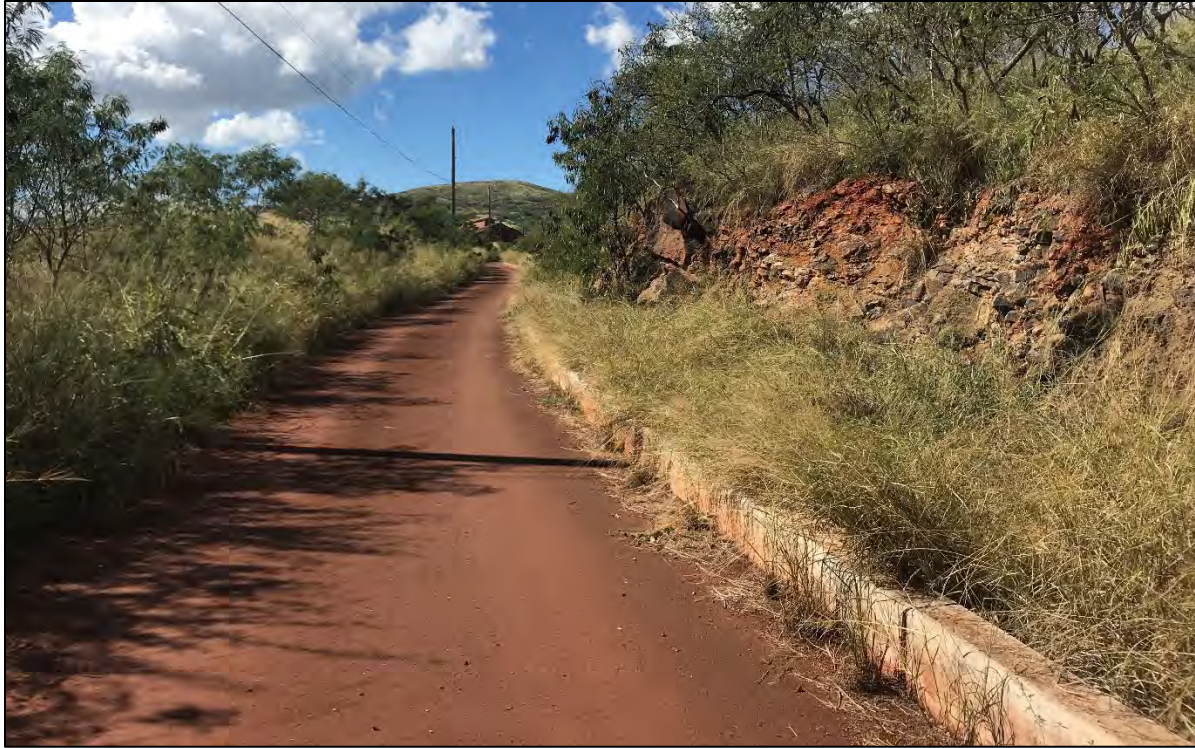
Figure 33. Access road encompassed within the project area, paved and lined with concrete curb, view to southwest
