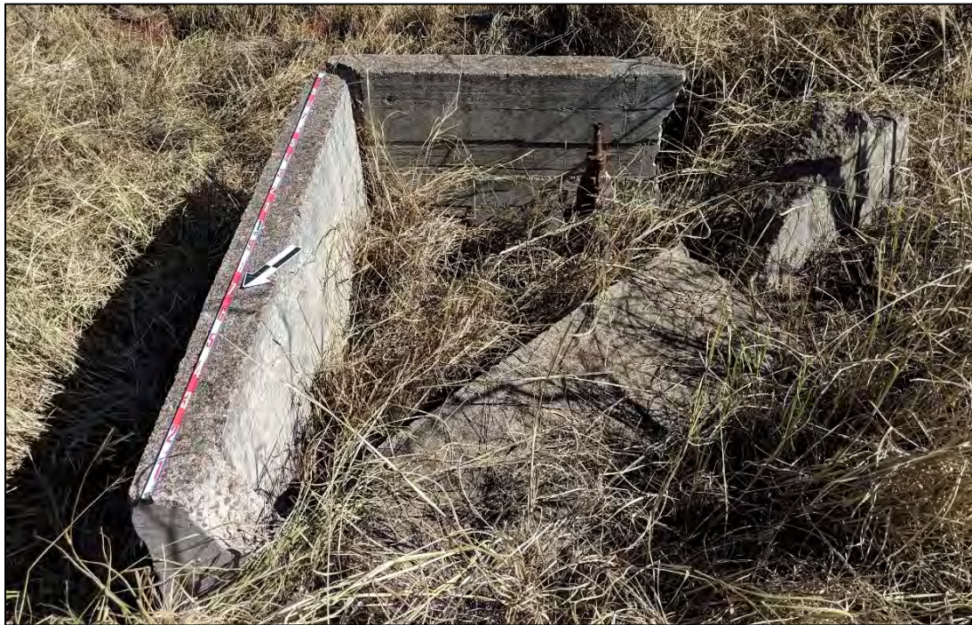
Figure 70. Collapsed walls with pipe, component of SIHP # 50-80-08-5593 Feature 2C, view to southeast
