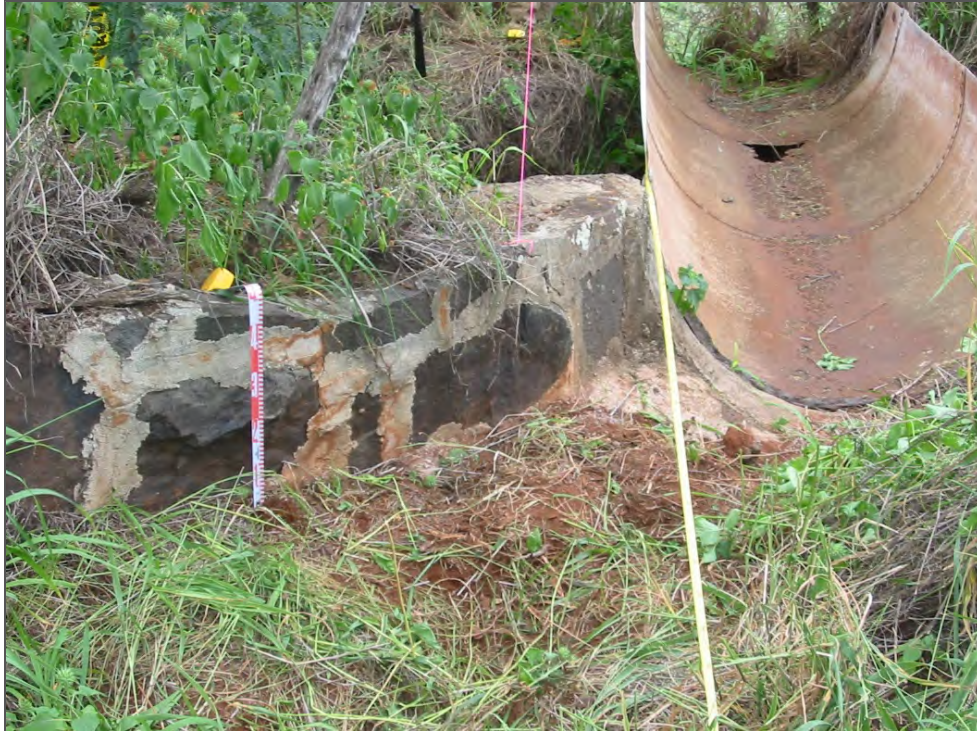
Figure 85. SIHP # 50-80-09-2268 Feature B, showing stone and mortar flume support foundation, view to north (Hunkin and Hammatt 2009:50)
