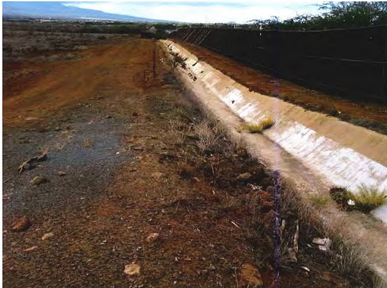
View of concrete drainage culvert that runs along the western boundary of the subject property and under Piilani Highway.
