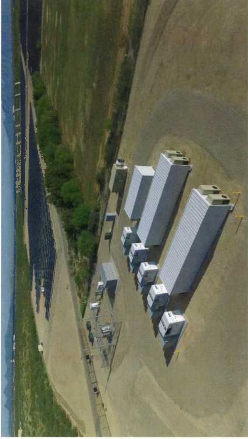
TEP Iron Horse Project (Battery integrator: Greensmith with EON)
