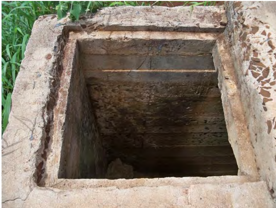
Figure 67. Overview Photograph of Embrasure with Concrete Encased Pipe to Right (top) View to West; Photograph of Access into Site 7883 (TS3) (bottom) View to West
