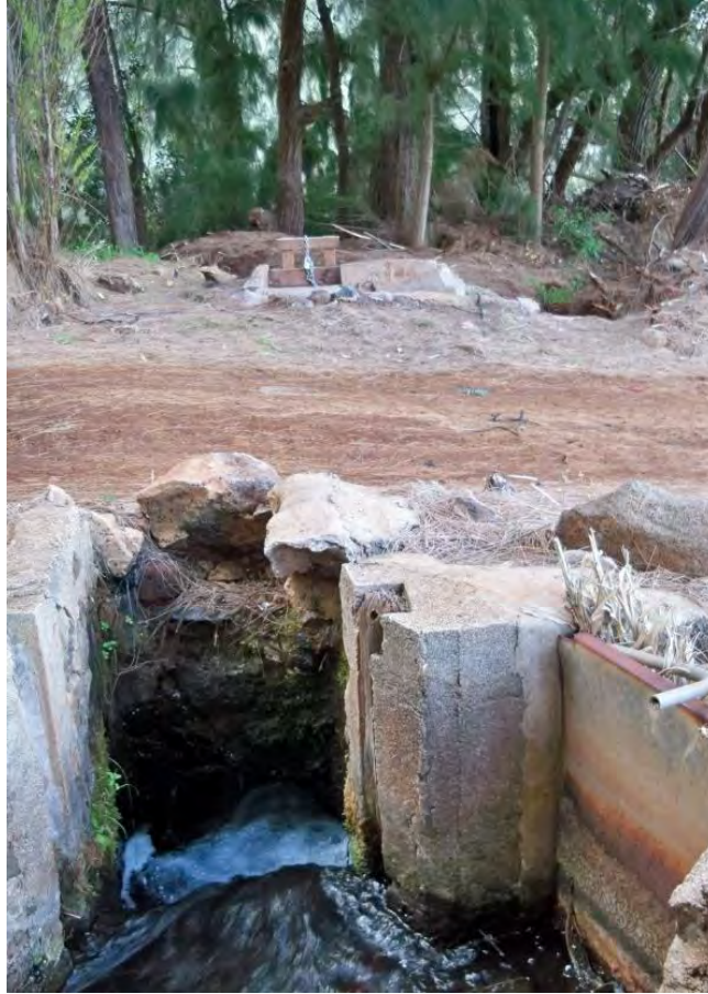
Figure 37. Site 7881 Feature 7 Sluice Gate in Foreground and Feature 8 Background (View to Northeast)
