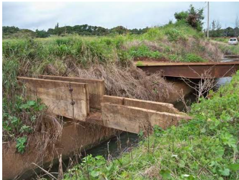
Figure 167. Overview Photograph of Second Bridge from the North, Metal Beam and Cement Construction (background), Older Drainage Culvert (foreground), View to Northeast
