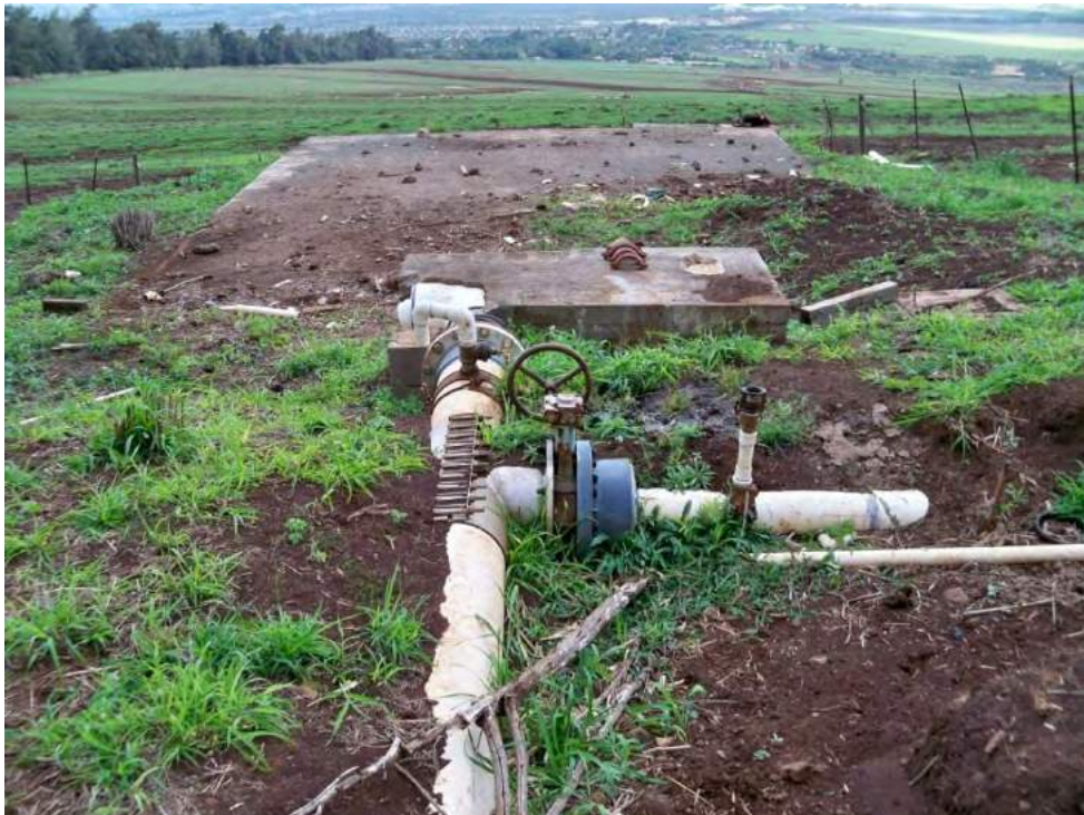
Figure 70. Overview Photograph of Site 7883 Feature 1 with Modern PVC Valves
