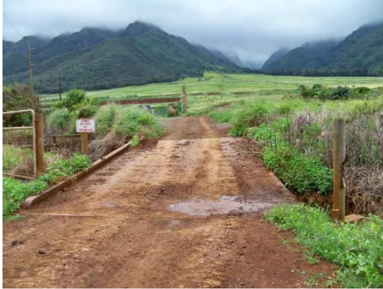
Figure 168. Photographic Overview Second Bridge, Metal Beam and Concrete Construction, View to West
