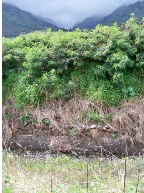
Figure 166. Overview Photograph of Site 5197 Waihe'e Ditch Showing Older Construction with Stacked Rock Atop the Concrete Lined Ditch (View of Western Side Wall
