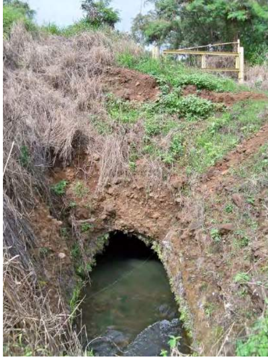
Figure 162. Overview Photograph Site 5197 Waihe'e Ditch Emerging from an Underground Culvert from the Northern Property Boundary, View to North
