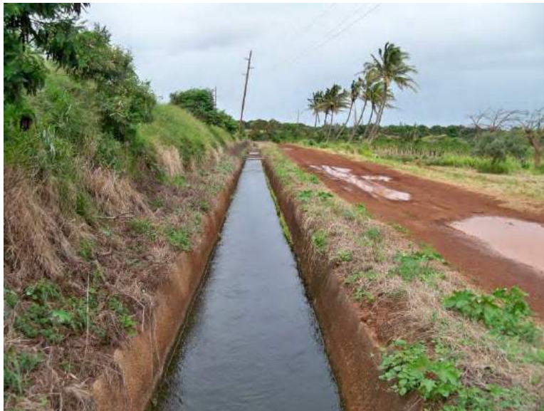
Figure 173. Overview Photograph of Site 5197 Waihe'e Ditch with Modern Concrete Lining, View to Northeast
