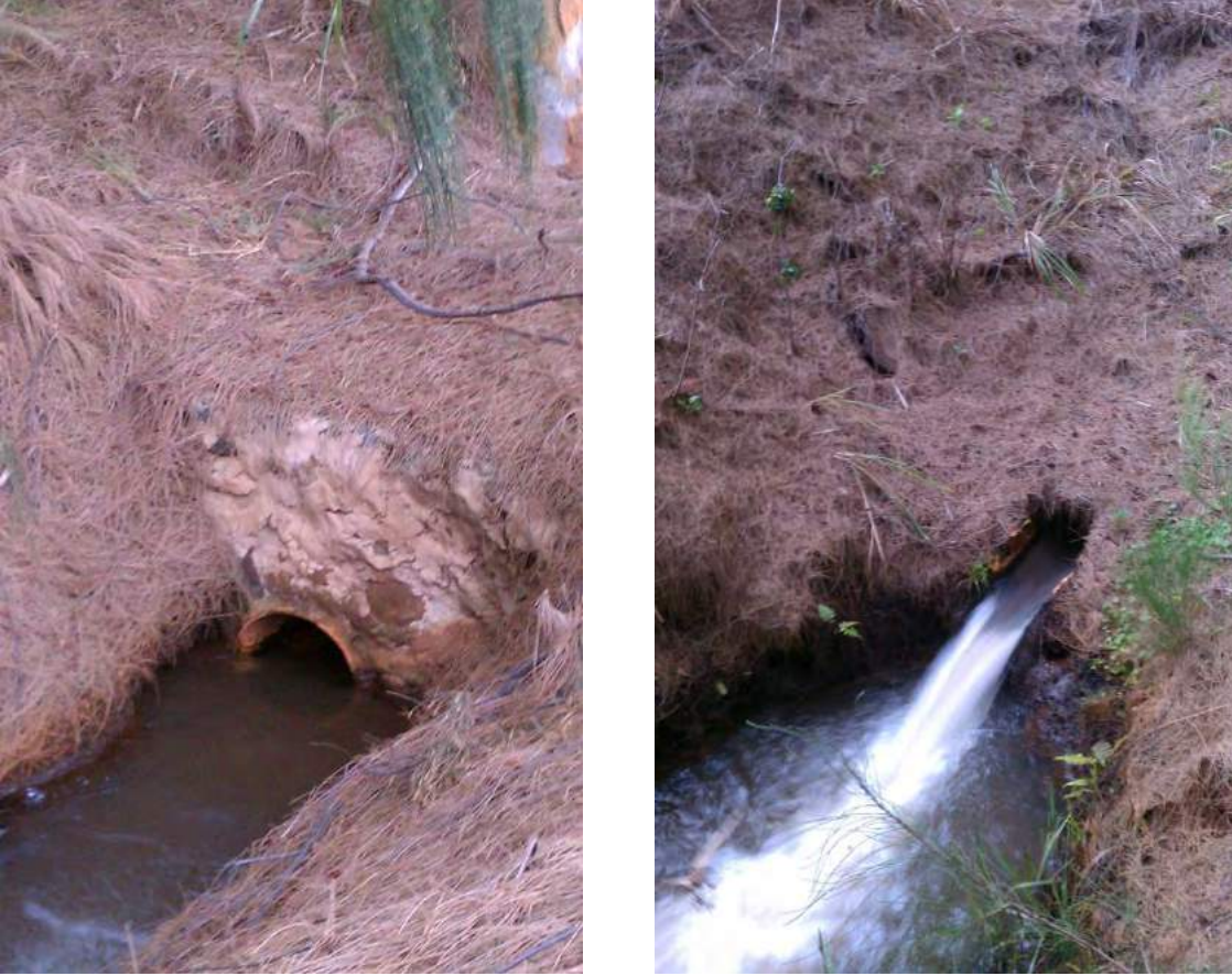
Figure 50. Photographs of Site 7881 Feature 15 In-take (View to East) left and Feature 15 Out-take View to West (right)
