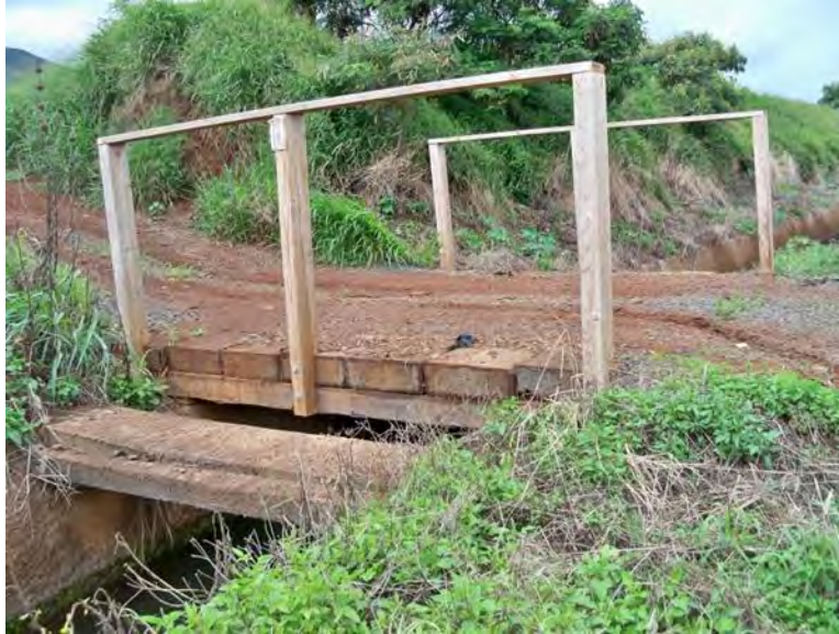
Figure 172. Overview Photograph of Fourth Bridge from North, West of Maui Tropical Plantation and Reservoir with Modern Wooden Construction, View to North
