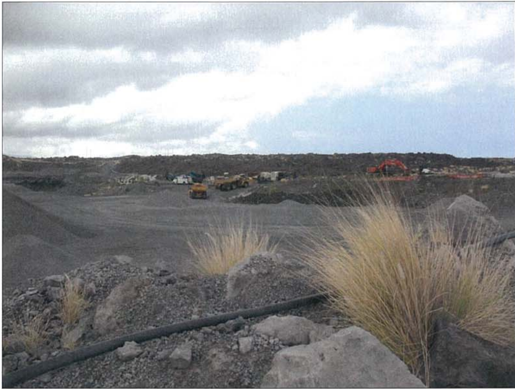
Figure 6. Mechanical quarrying activity within the current study area, view to the east.
